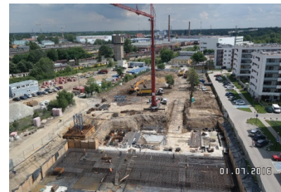
Apartamenty-Innova, Wroclaw (Building 6.3) No. of units: 120 units (8,335 sq. m). Breaking ground: April 2016. Progress to date: 3% (as at 30 June 2016). Delivery date: Q1 2018. On sale since: June 2016 (15% presold as at 30 June 2016).
