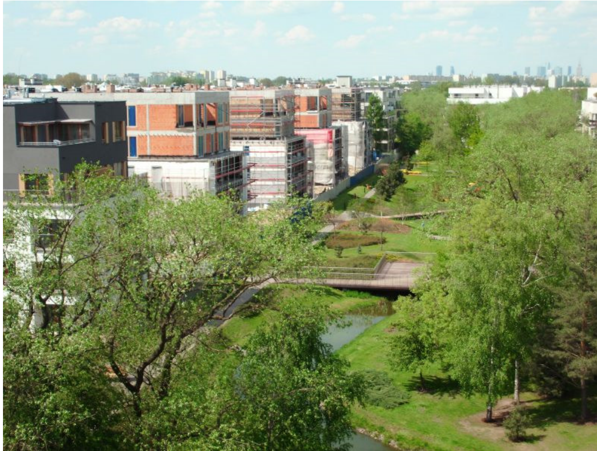
Construction of buildings C2 on the left bank of the central lake in Ostoja-Wilanów, Warsaw (May 2016).
